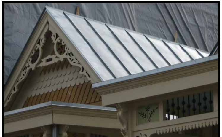
YES —This metal standing seam roof was designed to match historic profiles in crimping and spacing. This type of roof would be appropriate if a metal roof was original to the dwelling and removed at a later date.
