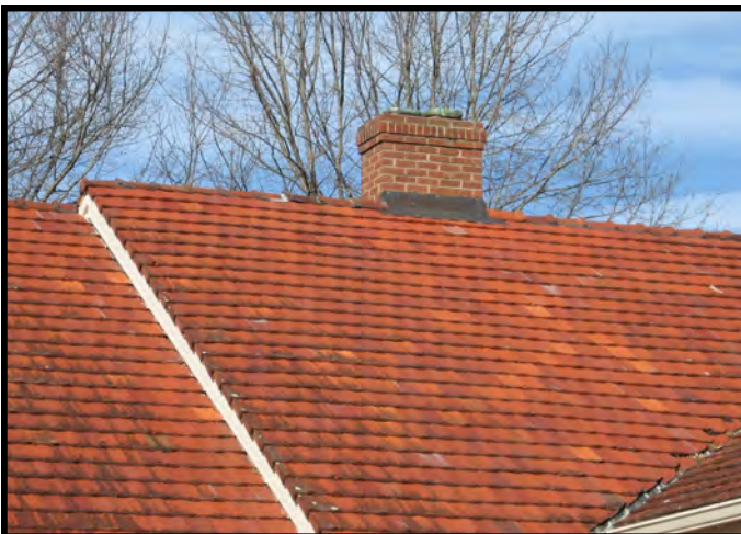
Clay tile is a long-lasting and durable roof material applied to early twentieth century houses (840 Jackson Street, SE).
