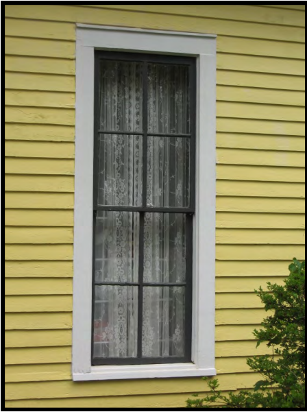
Some of the oldest windows in the overlay districts are four-over-four wood sash design (501 Line Street, NE).
