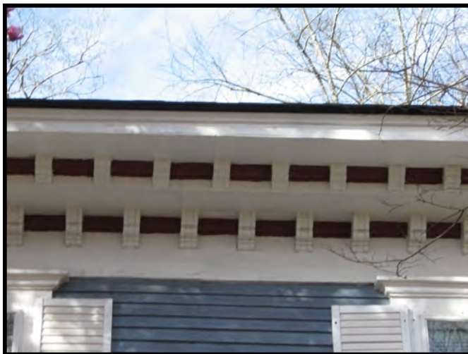
Small eave brackets are at the roofline of the Italianate dwelling at 636 Johnston Street, SE.
