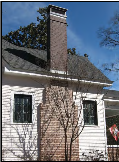
Preserve and maintain exterior wall brick chimneys. Some chimneys have particular detailing such as stepped shoulders and decorative brick courses (701 Line Street, NE).
