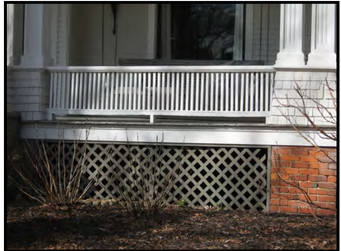
Appropriately designed and placed lattice panels between the porch foundation piers at 650 Jackson Street, SE.
