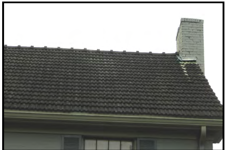
Cement tile is another twentieth century roof material which should be preserved and maintained as long as possible (604 Line Street, NE).
