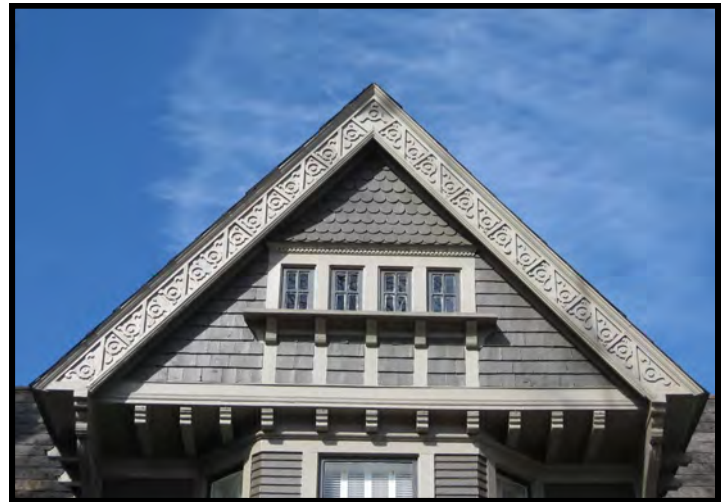
The dwelling at 616 Sherman Street, NE, features a variety of vergeboard trim and wood shingles in its gable.
