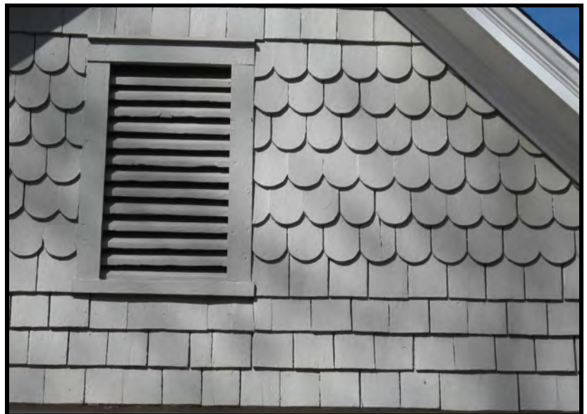
Some gable fields display both square and fishscale shingles as at 403 Canal Street, NE.
