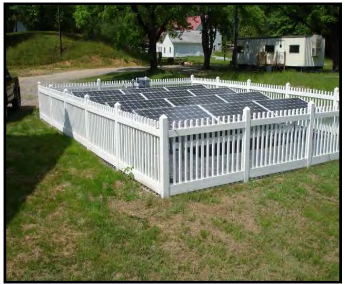
YES —Free standing solar panels may also be sited and screened in rear yards.
