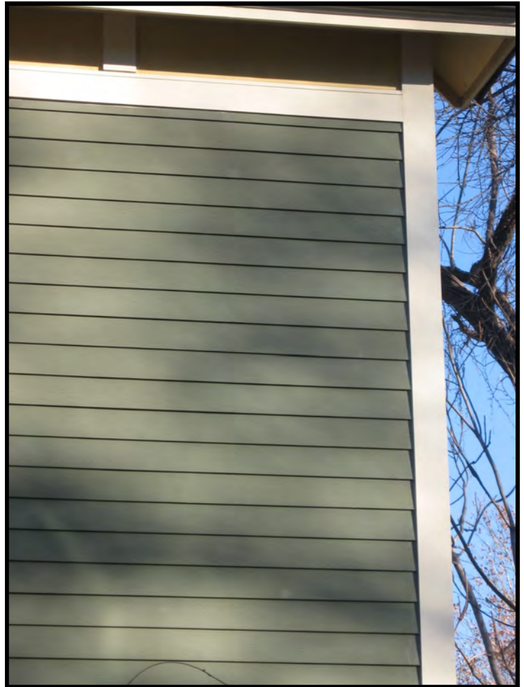
Cementitious siding may be an appropriate alternative siding material in some cases if it has the appearance of historic wood siding.
