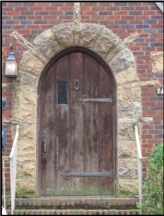
The rounded arch door and stone surround at 422 Oak Street, NE, help define the dwelling's Tudor Revival style.
