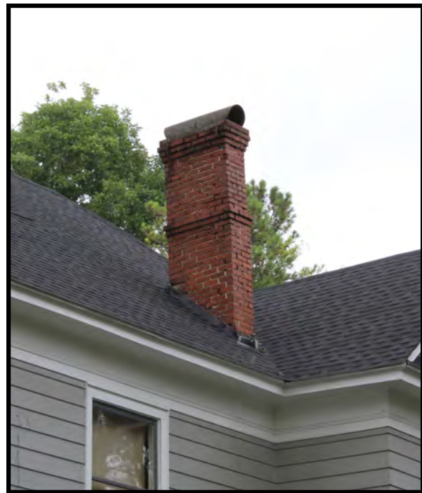
Preserve and maintain decorative chimneys, such as this distinctive design at 315 Lafayette Street, NE.
