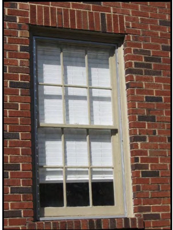
Colonial Revival and related styles were often built with six-over-six wood sash windows (621 Canal Street, NE).
